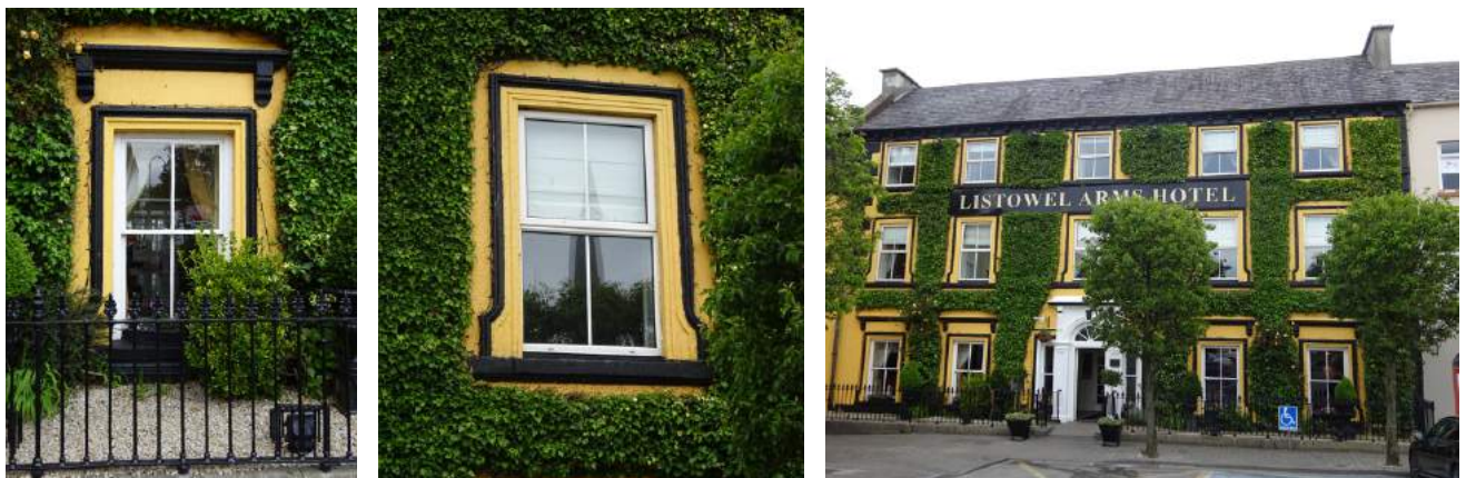
A comparison of the ground floor timber sash windows (far left) and the first and second floor outward opening uPVC windows (middle) to the Listowel Arms Hotel demonstrates the differing characteristics of the two materials and opening arrangements and the impact that can have on the entire facade (right). The uPVC windows, with false mullions, lack depth and material character.
