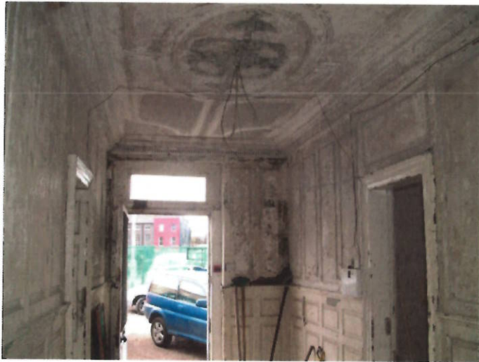
Picture on the left is the hall before conservation works and pictures below show the hall following completion of conservation works
