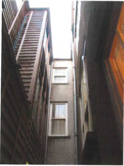
Pictures to left and below show new extension to rear of protected structure to accommodate secondary access and services. Contemporary design and finish works well.
